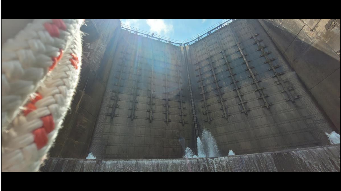
Lock 4 double doors – this is the photo which Bill was framing on the last slide
